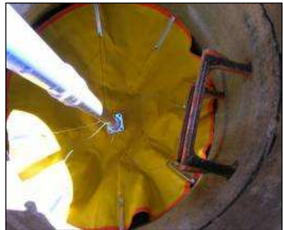
Debris Dam Placed in Manhole
